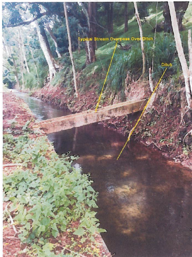
Photo 2 (below): Typical "stream overpass" intended to prevent the ditch from intercepting a stream
