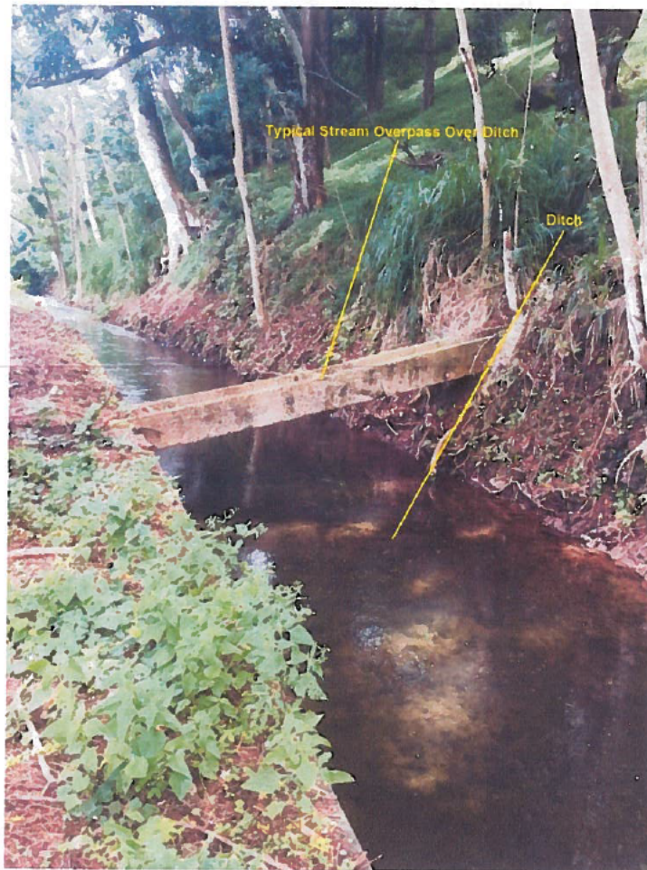
Photo 6 (below): Typical “stream overpass” intended to prevent the ditch from intercepting a stream
