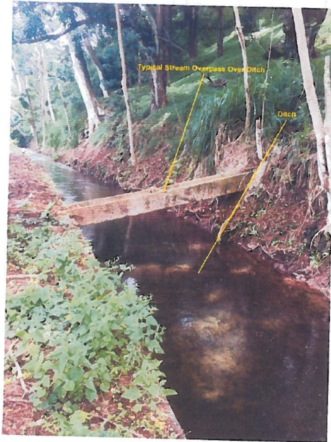
Photo 14 (above): Typical “stream overpass” intended to prevent the ditch from intercepting a stream
